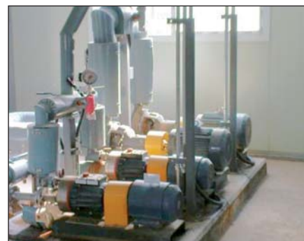
PHOTO 1. Hydra-Cell G25 seal-less pumps at Seonam.
