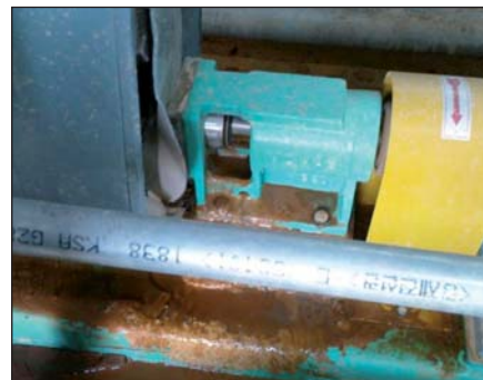
PHOTO 2. Abrasives were a problem for screw pumps.
